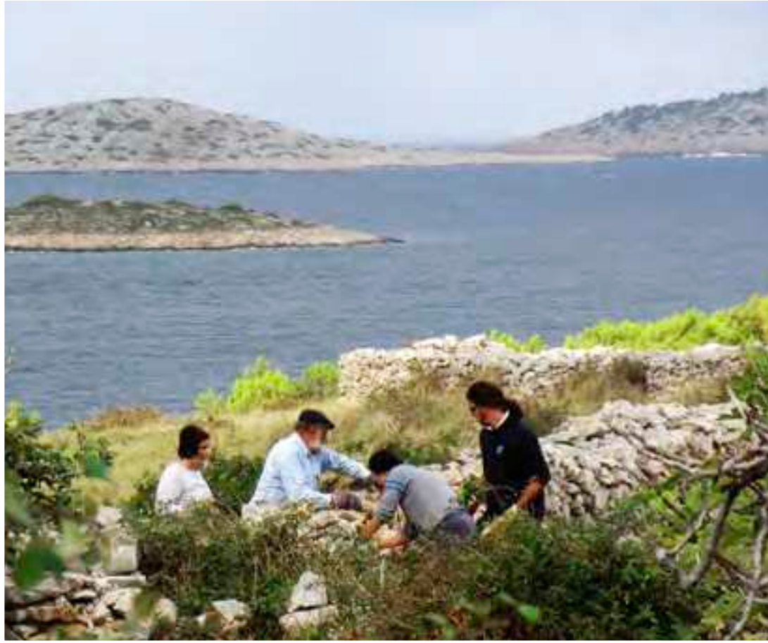
Kornati: Building and renewal of dry-stone walls, 2015. Photo by Vilma Stopfer, © Association 4 grada Dragodid.
